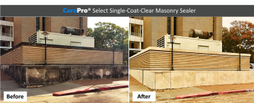
Figure 3] Sandstone facades severely soiled from extensive fungal and lichen growth remain in pristine condition 6 months after application of CaraPro® Select Single-Coat-Clear Masonry Sealer.
